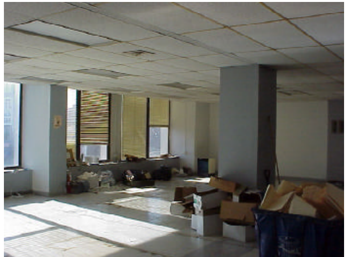
The facilities management team scouted out locations across Manhattan and selected this office space at 215 West 125th Street in addition to locations on 91st Street in Queens and Livingston Street in Brooklyn. The above photo shows the Manhattan office prior to construction.
